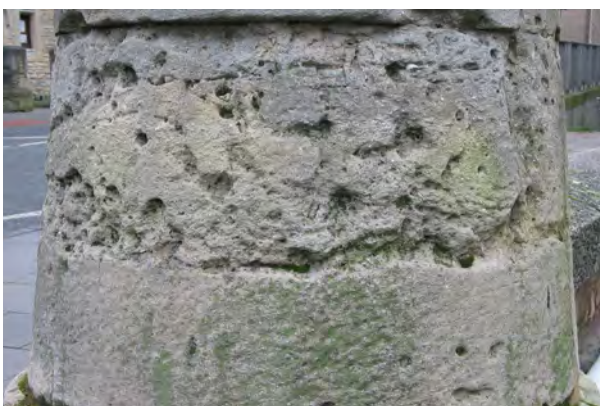
Fig. 5a Differential weathering of limestones that have local patches of micrite with high microporosity in them. 5a, micrite-rich burrows in (probable) Headington Stone weathering out to give cavernous texture. 5b, micrite-rich laminae in Milton Stone.
